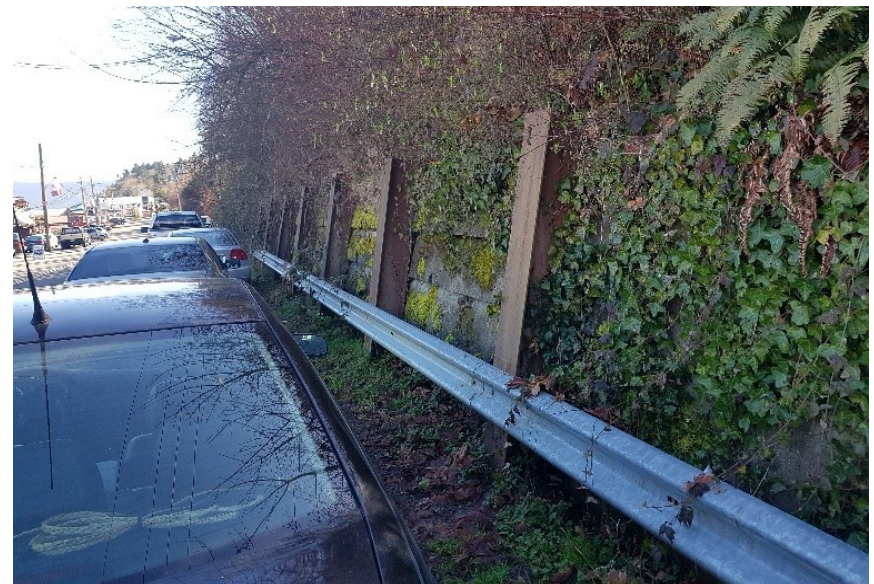
Photo 5: View of Cowichan Bay Road looking east with upslope soldier pile wall.
