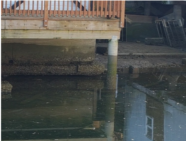
Photo 1: View of existing structure founded on spread footing with deck founded on piles.
