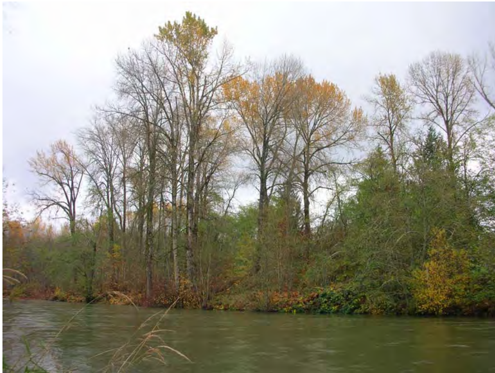
Photo B.12. Lateral view of south side dike at km 5.7 adjacent to the right bank shoreline where proposed dike maintenance will require removal of vegetation along both sideslopes. Riparian vegetation is currently providing overhanging cover, refuge and food supply to salmonids. Dike maintenance activities will require consultation with FOC and likely require details of the proposed maintenance along with a compensation plan and monitoring plan (Nov 2008).
